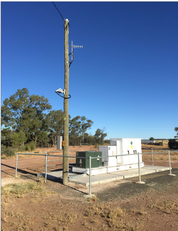
An installed Grid Utility Support System unit in the field.
