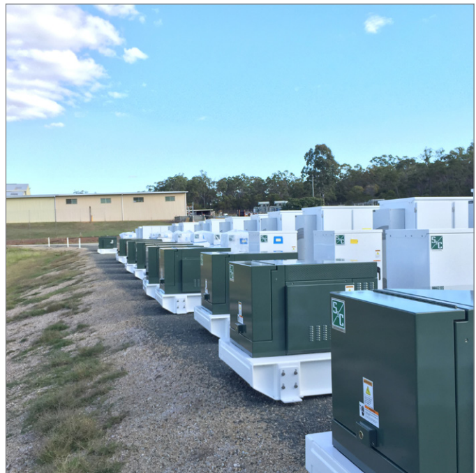
Delivery of the Grid Utility Support System units to Ergon's stock yard.
