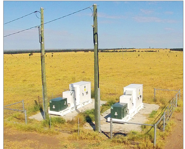
Twin Grid Utility Support System units providing extra support along a SWER line.
